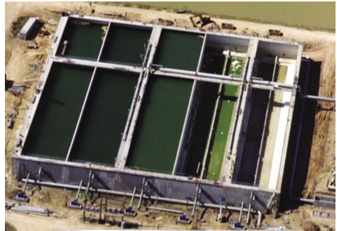
Fig. 5: This open-top post-tensioned aeration was built for the Bayport Wastewater Treatment Plant in Pasadena, TX
