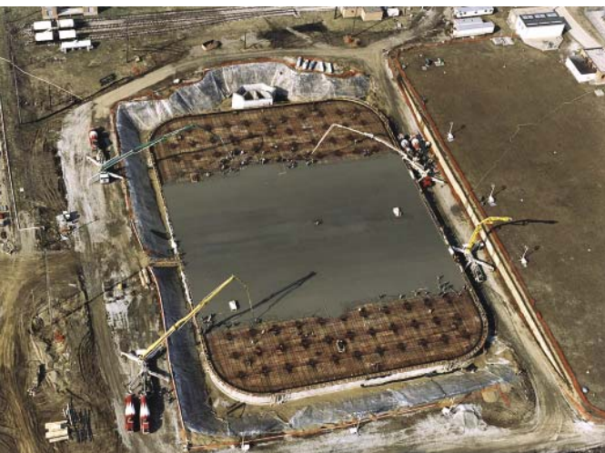
Fig. 3: A rectangular PT concrete tank with rounded corners at the White River Water Treatment Facility in Indiana
