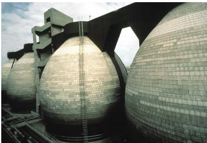
Fig. 6: Terminal Island egg-shaped digesters built in Los Angeles, CA (Photo courtesy of VSL)
