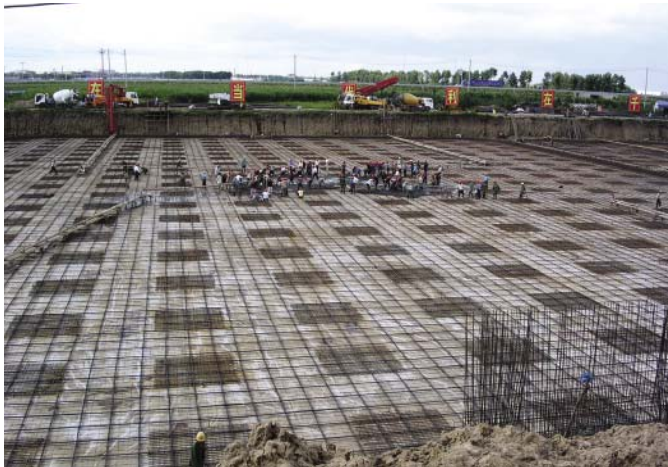
Fig. 4: A rectangular PT concrete tank with rounded corners under construction in Harbin, China
